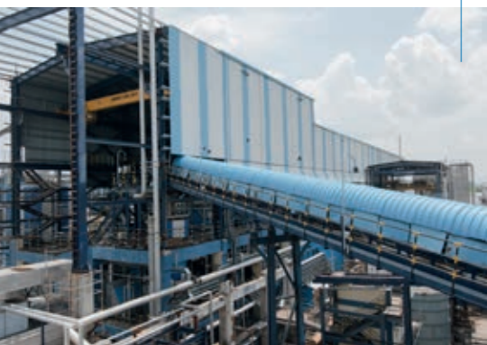
Conveyor feeding chips into the mill.
